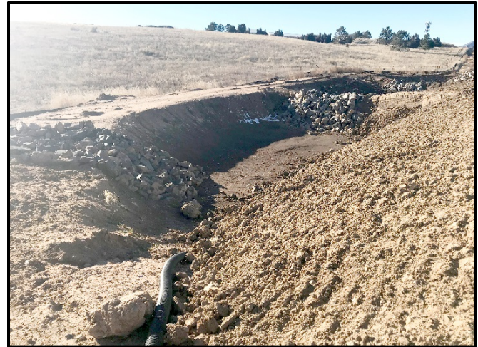
Sediment Trap downstream of rock check dams
